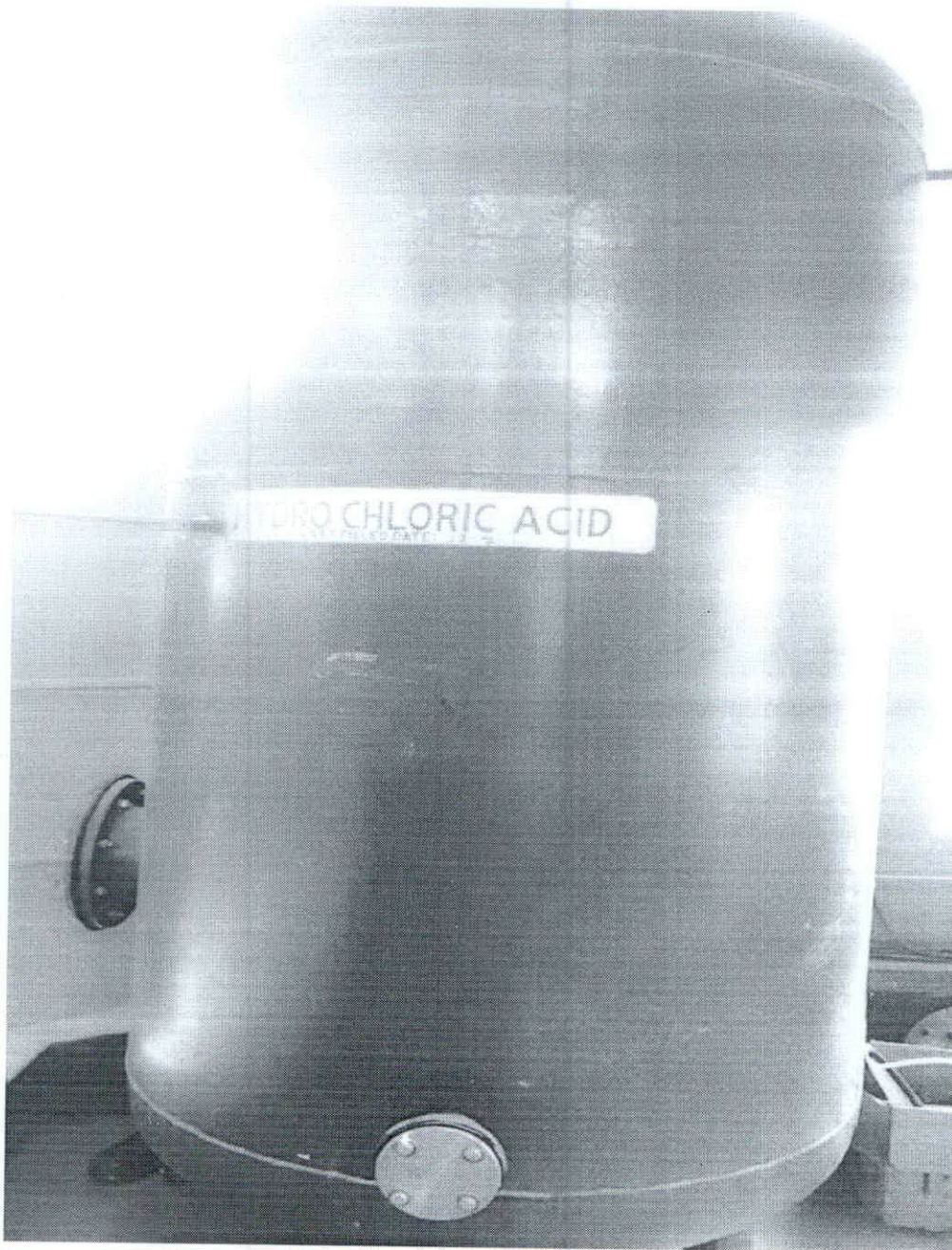
Fig 1.9 Hydrochloric Acid for Disinfection
