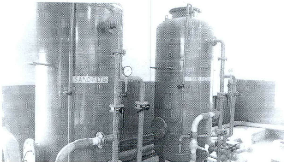
Fig 1.7 Sand Filter Units
